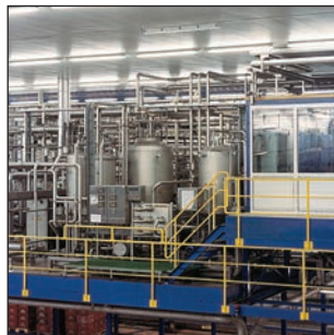
Technical rooms • Chemicals • High temperature • Vibrations • Chloric gases
